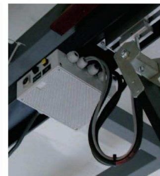
Terminal box (ceiling)
